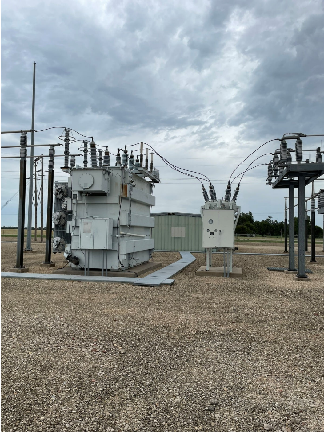
Figure 1: Seward 115kV/69kV Transformer and Cable Trench
